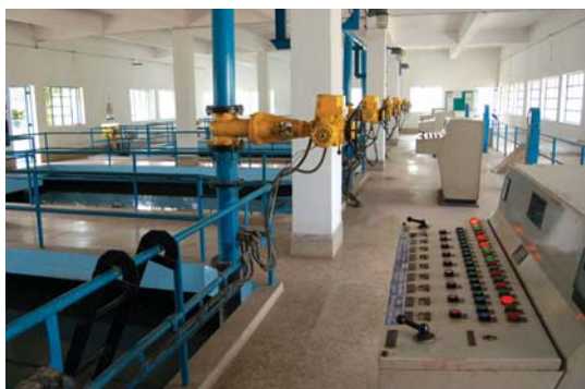
Jusco's state-of-the-art water treatment plant in Jamshedpur
