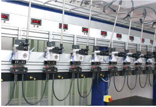
The new electricity meters
